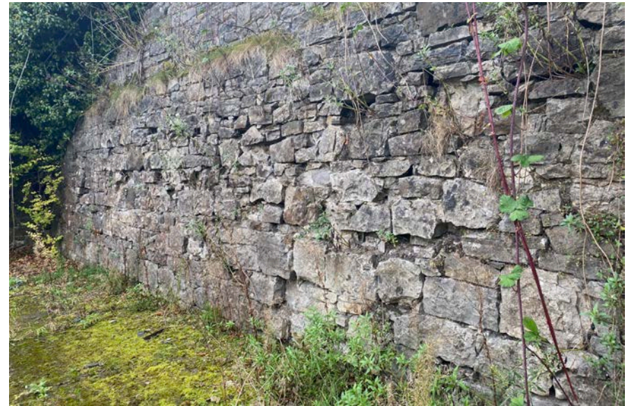
52. Detail of stonework in poor condition to base of bastion.
