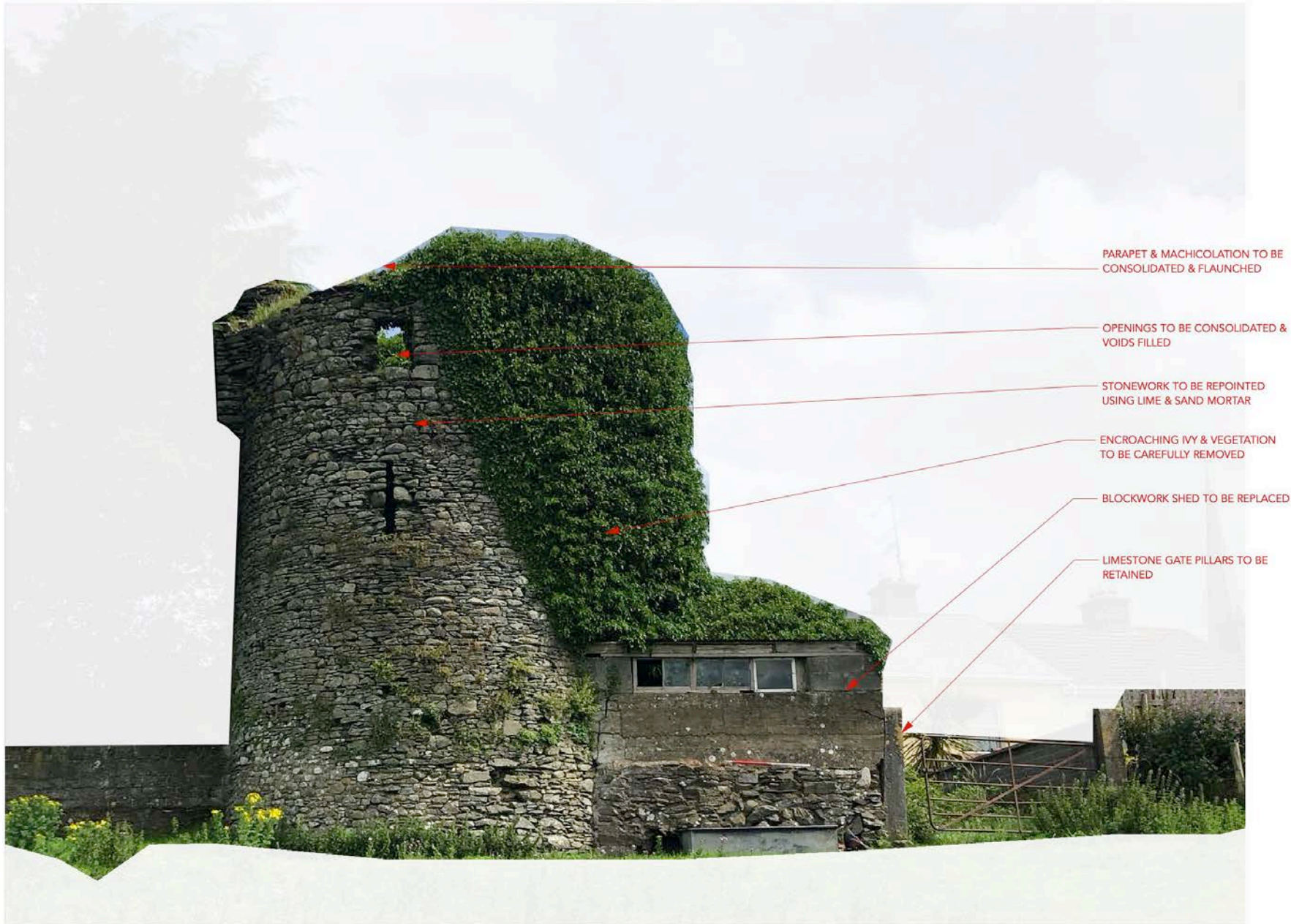
43: View of defects to mural tower.
