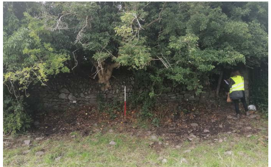
22: View of stone facing in bank with heavy vegetation growth.
