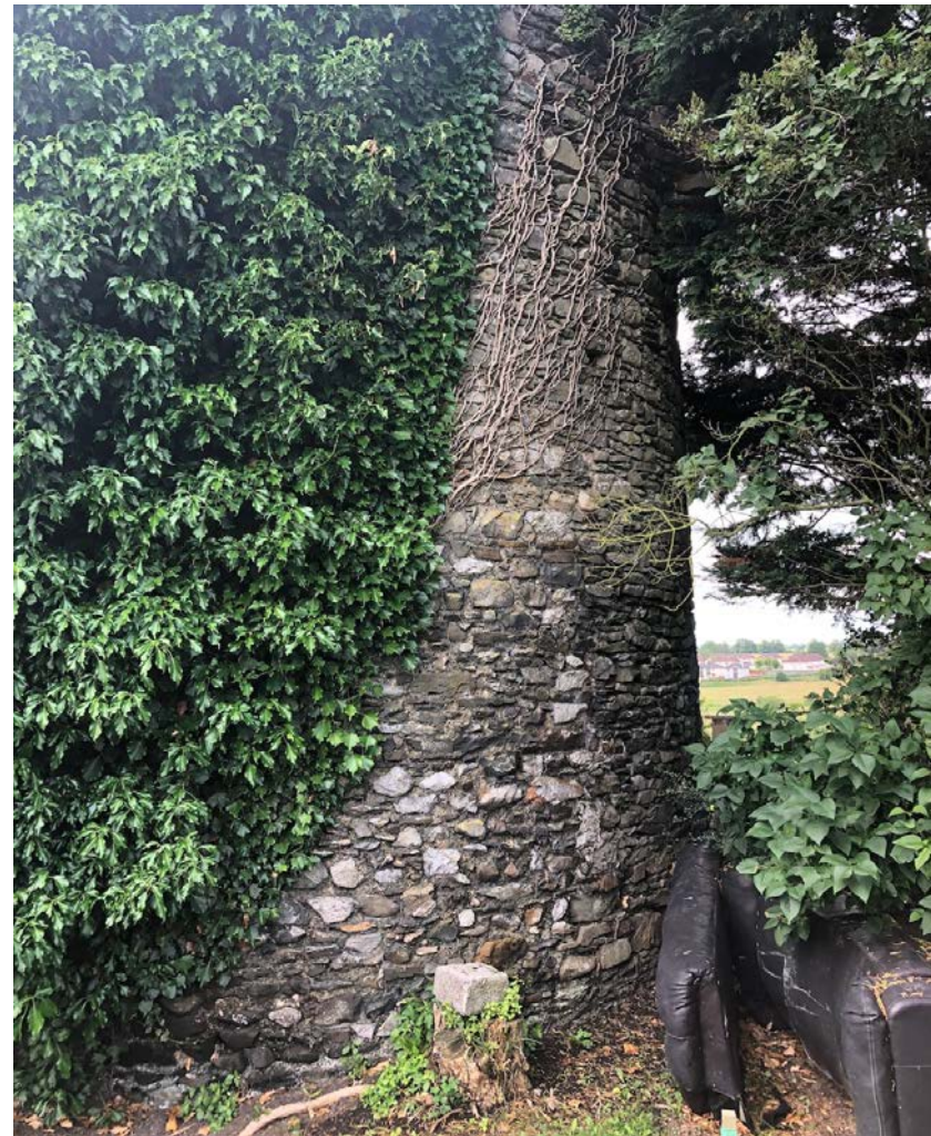
30: Detail showing exposed side with no visible evidence of wall scar.
