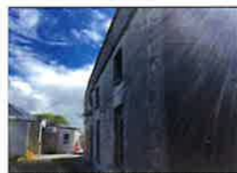
Photo - 11 Note: Structural bulge to front wall due to
