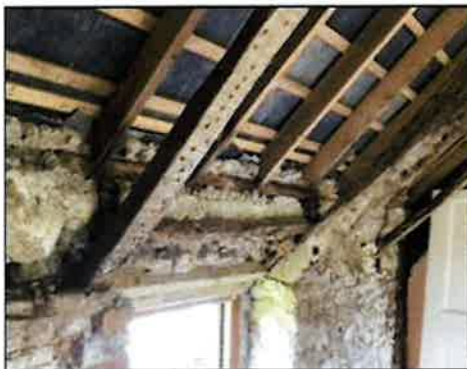
Photo - 44 Note - rotten roof timbers and window heads throughout.
