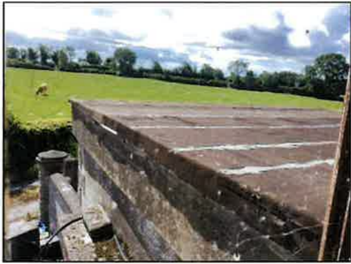
Photo - 6 Flat Roof to rear Kitchen extension requires replacing to a new Warm Roof system
