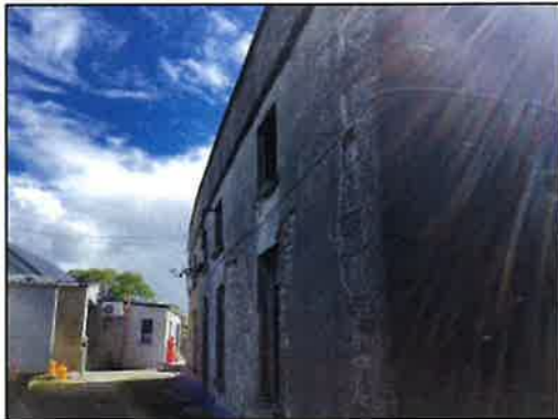
Photo - 11 Note - structural bulge to front wall due to deteriorated roof valley.
