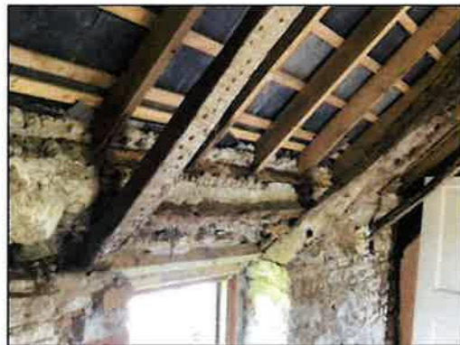
Photo - 44 Note - rotten roof timbers and window heads throughout.
