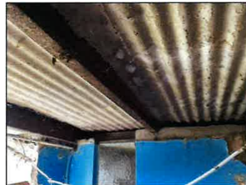
Photo - 53 Incorrect reinforced concrete detail therefore must be removed as structurally unsound and dangerous.
