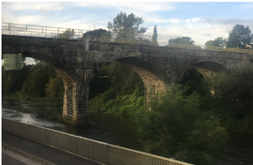
Seven arch railway viaduct over river c. 1849 of rock faced rusticated limestone .
