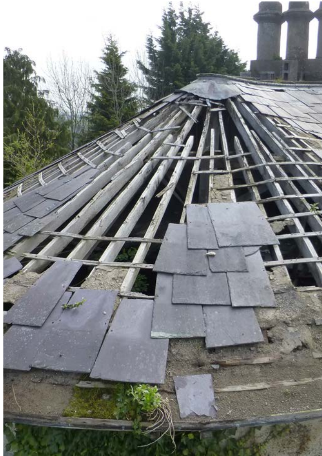
Poor roof condition.
