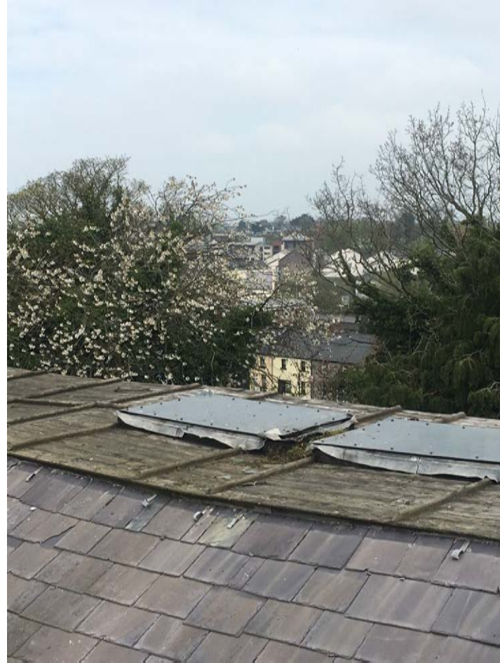
Two openings in the roof that would have accommodated lanterns in the past .
